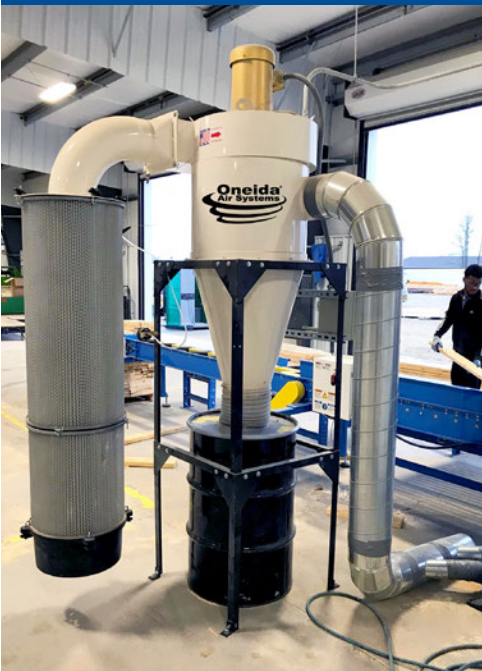
Oneida Air Systems' High Vacuum dust collector connected to a MiTek Matchpoint blade saw at one of Carter Lumber's manufacturing sites.
